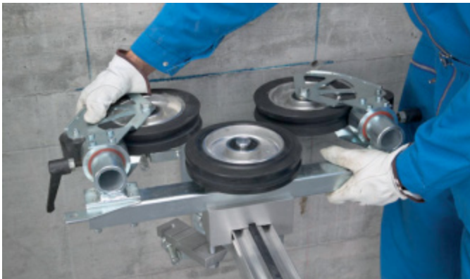
Bring the pulley crossbar into position (note the distance from the wall).
